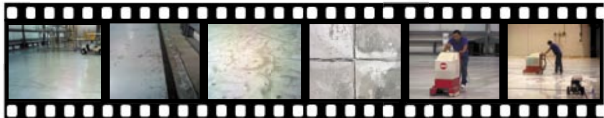
Conditions at Project Start
