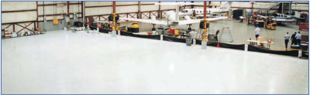
Epoxy Primer (E31-1202-64) application / an important consideration was to keep the other half operational as much as possible.
