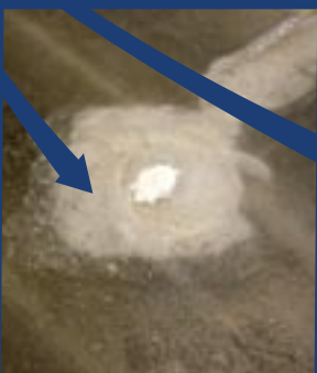
Holes diamond ground / filled with E31-1204 then sanded flush to the floor
