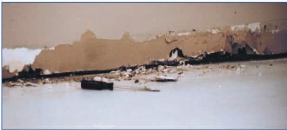
Entry way to shop / conditions after tile removed
