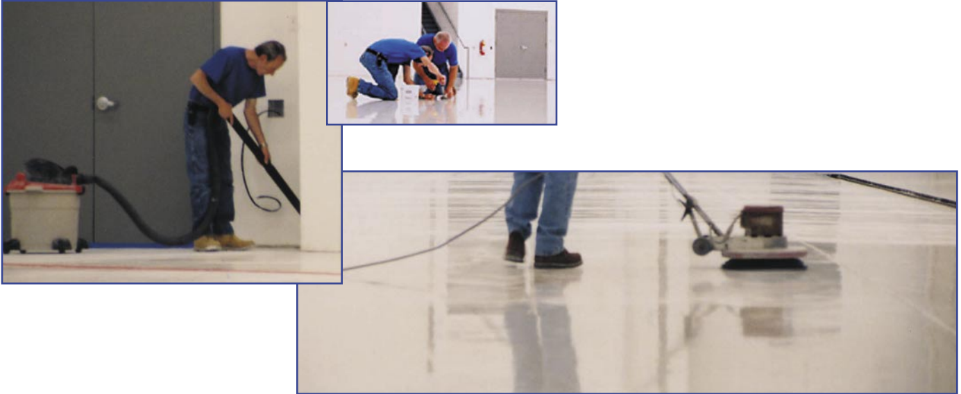
100% solid epoxy overlayment applied ( E31-1202 ) and sanding started [preparation before high performance urethane topcoat application ( U31-1201 )]
