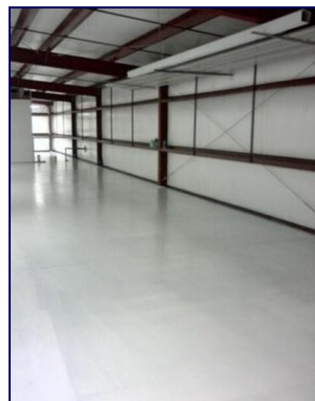
E31-1202-64 epoxy primer applied to back rooms of hangar ("lean to" building)
