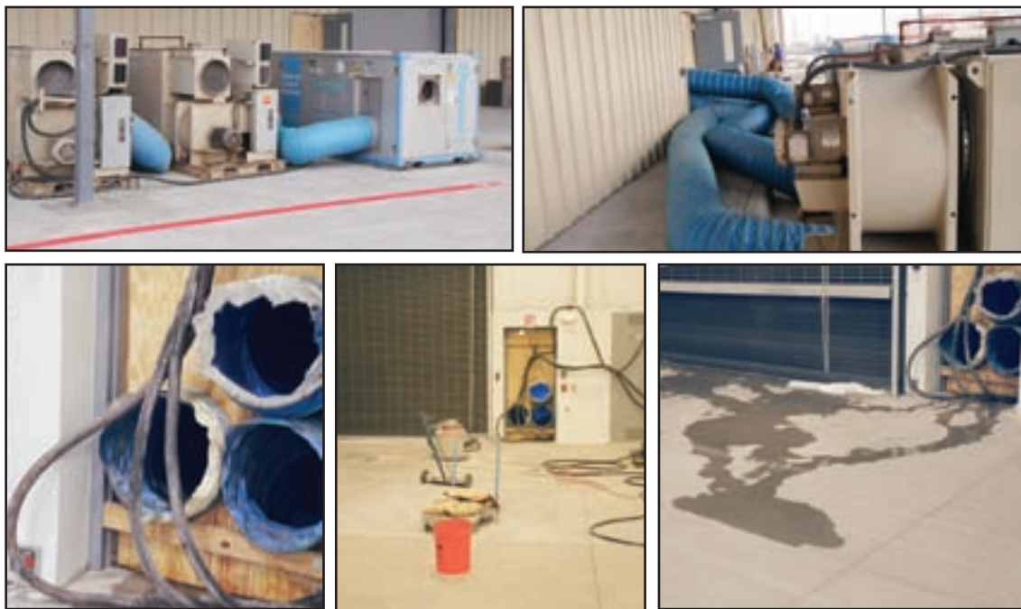
Moisture Control Equipment (Three Units) Pumping in Dry, 112°F Air For Two (2) Weeks
