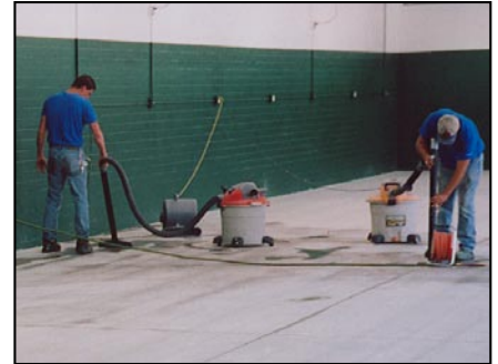
Vacuuming of accidental water release - project delayed for one day.
