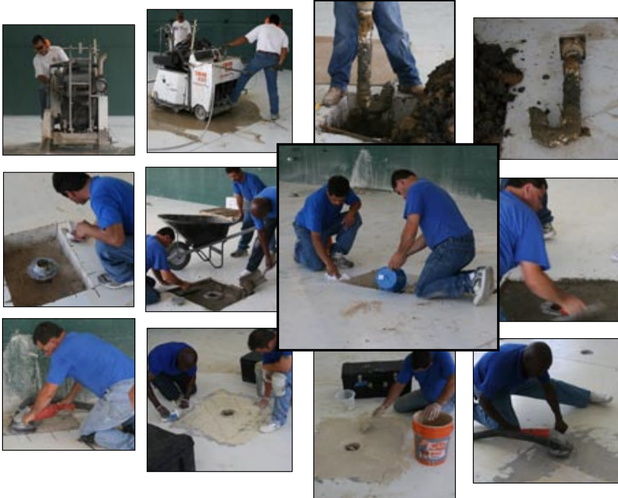
These photographs display the cutting, breaking-out process, and the placing of new drains.
