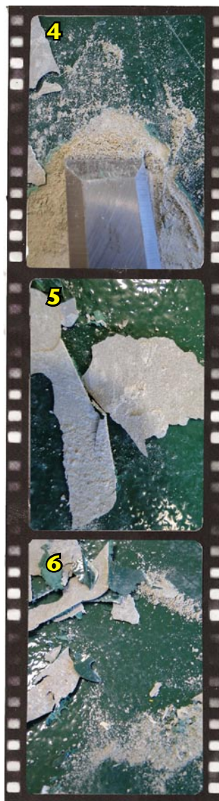
Photographs (4-6) show concrete bonding to coating (which is good), therefore leading to questions of the integrity of the concrete immediately below the coating failure.
