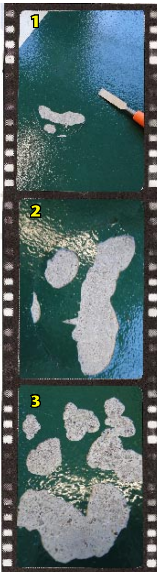
Photographs (1-3) show peeled areas during initial “exploratory preparation” stage.
